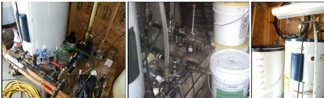
Modified water heater for Biodiesel production found in a Salem Township mobile home park.
